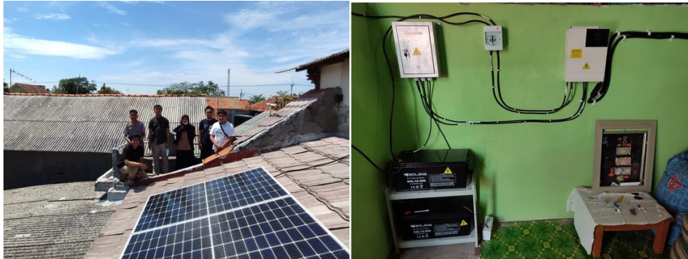
Figure 6. PV panels installed on the roof of SME's house and an electrical system that has been installed in a room dedicated to solar power system.
