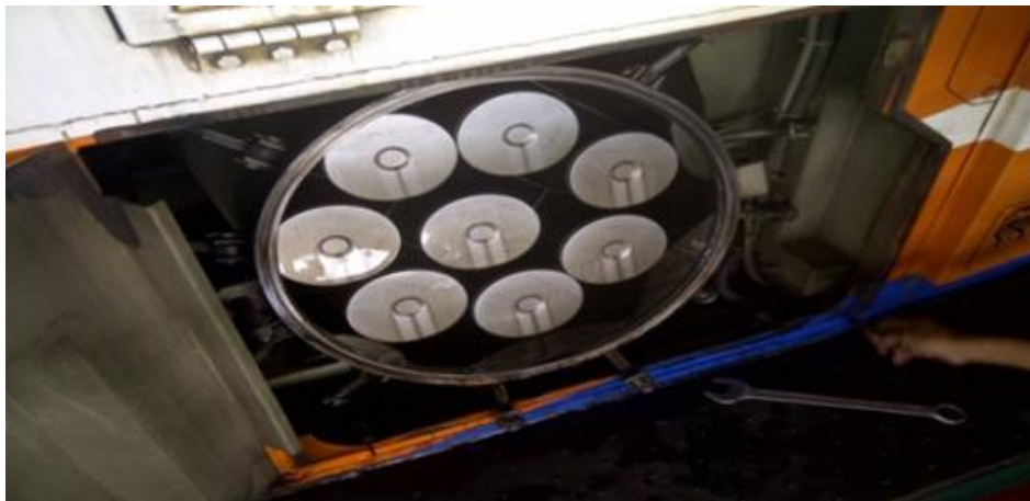
Gambar 14. Lube Oil Filter
